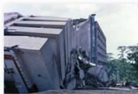
Earthquake-induced damage during 1995 Kobe Earthquake
